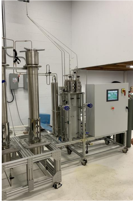
Figure 2. AE-100-series high-pressure pilot system: processing columns, separator train, and PLC/HMI control cabinet.
